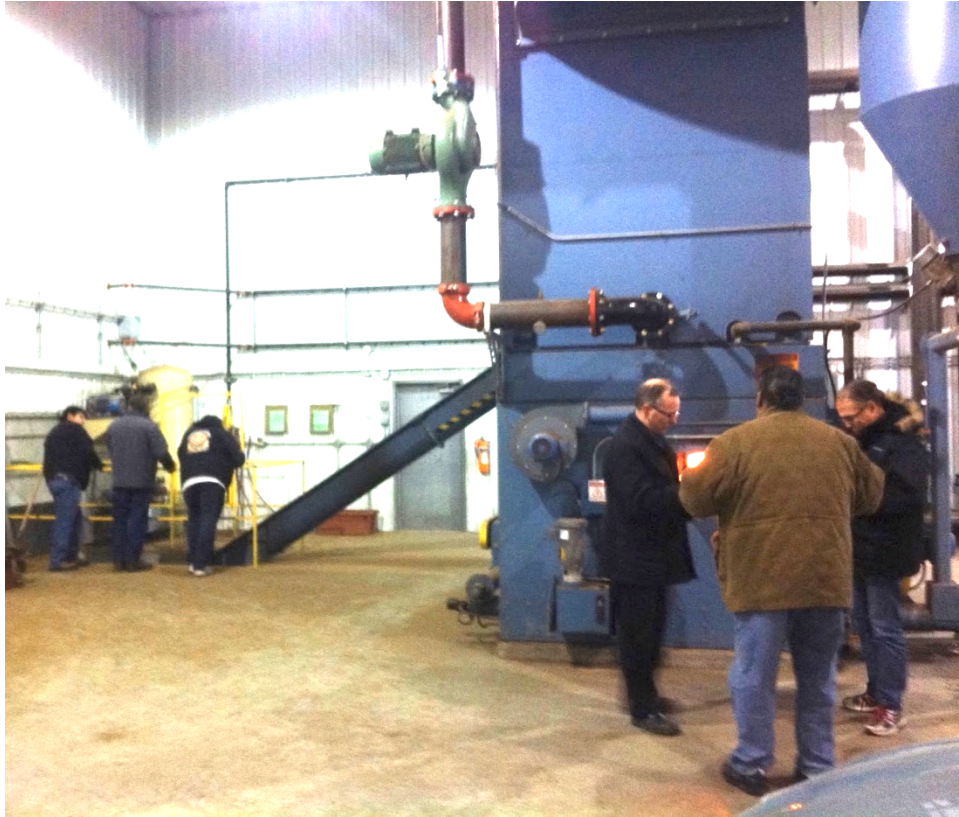
Figure 73. Auger Sending Fuel Into Boiler
