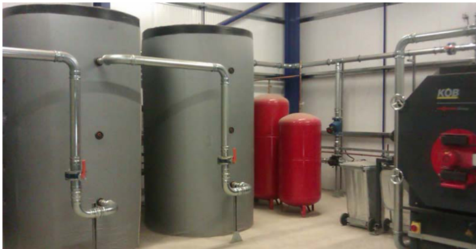
Figure 74. Indoor Buffer Tanks
