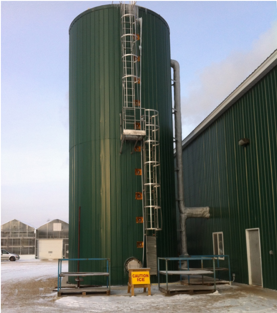
Figure 75. Outdoor Buffer Tank
